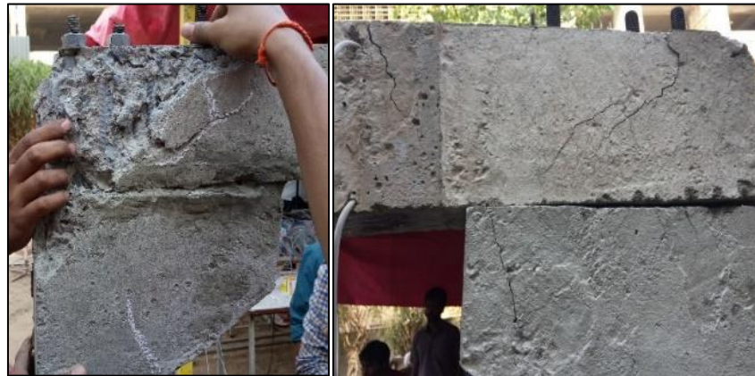
(a) Nearer beam column junction (b) Far end beam column junction
