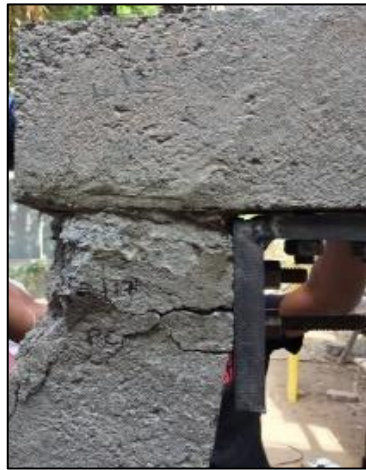
(a) Nearer beam column junction
